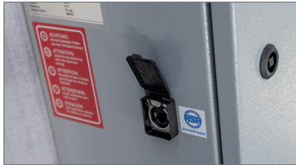
External data interface, e.g. for WiFi access point
