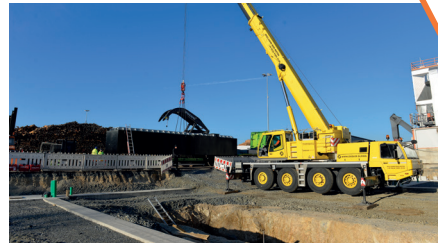
The TRUCKBAY is lifted in one piece with a crane to its destination.
